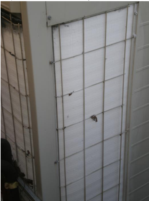
Fig 1 Frost build-up on air source heat pump evaporator
