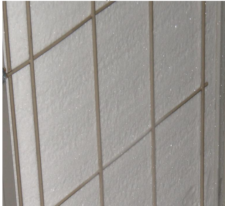
Fig. 2 Close up of evaporator fins showing airflow blocked by ice
